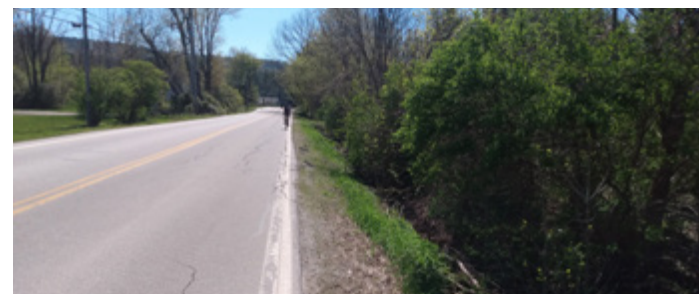
Steep side-slopes line the entirety of Route 30 between New England Slate and Furnace Street.
