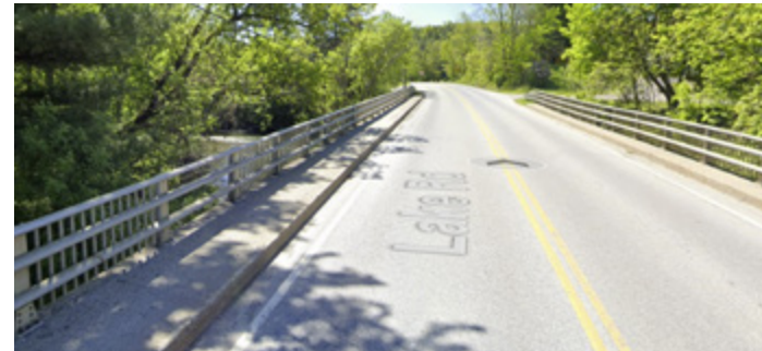
A 5 foot wide sidewalk is present on the eastern side of the Poultney River Bridge.
